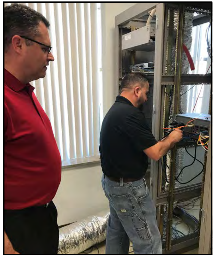
As Craig Ricke watches, a OneNet technician is installing equipment paid for by a grant from the National Science Foundation (NSF) that will give NWOSU a 100Gbps connection to the OneOklahoma Friction Free Network (OFFN). Work continues to make this service possible on our campus.
